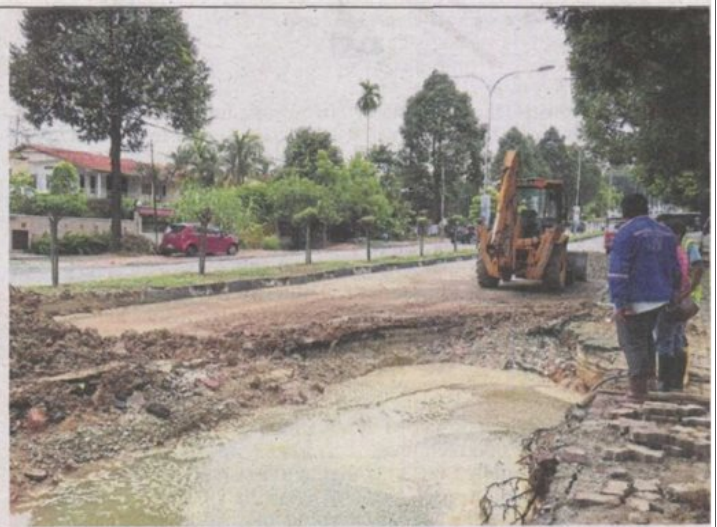
Contractors seen repairing the burst pipe along Jalan 17/1 in Section 17, Petaling Jaya. According to Syabas, water supply is expected to resume at 6am today. — Photos: JAROD LIM/The Star
